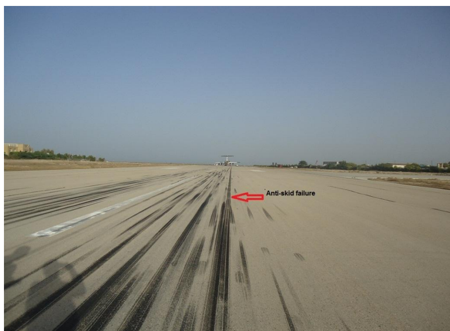
Signs of anti-skid failure
