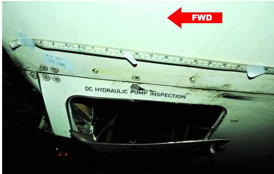
Figure 5: The hole on STA 15589
